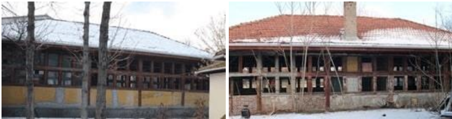
Figure 4. Images of the north (on the left) and south (on the right) façades of the building (Ankara Metropolitan Municipality Culture and Nature Department Archive, 2023)
