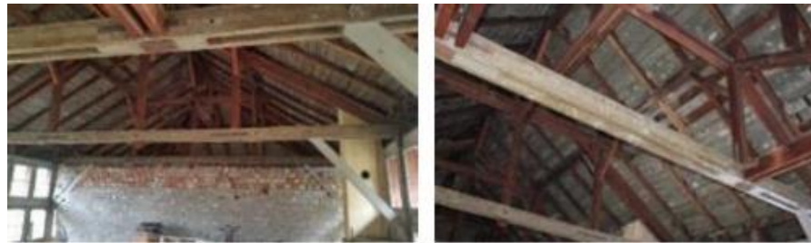
Figure 7. Wooden trusses and beams on the roof of the registered structure (Ankara Metropolitan Municipality Culture and Nature Department Archive, 2023)
