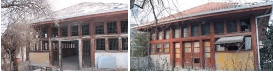
Figure 3. Images of the west (on the left) and east (on the right) façades of the building (Ankara Metropolitan Municipality Culture and Nature Department Archive, 2023)
