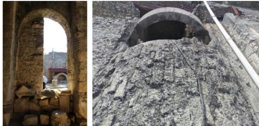
Figure 19. The outer narthex that closes off the western corridor arch and its collapsed vault (AMoCT-PR-4)
