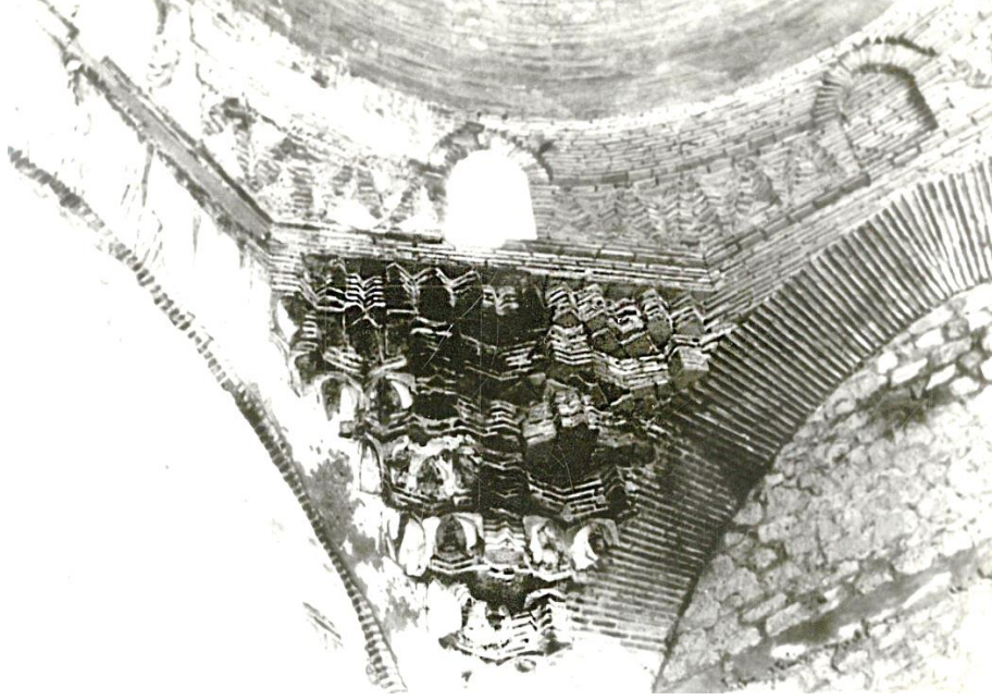
Figure 18. Muqarnas pendentive at Karacabey Mosque. Remnants of plaster details over muqarnas are remarkable. Source: Hassa Mimarlik Archive.
