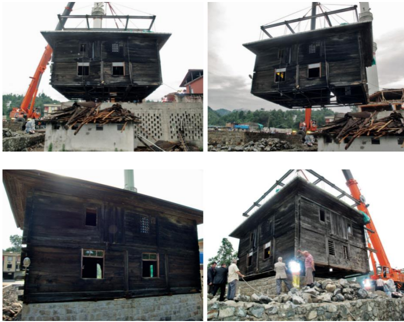
Figure 52., 53., 54., 55. Relocating the mosque in its new position by means of a crane (Sav, 2012)
