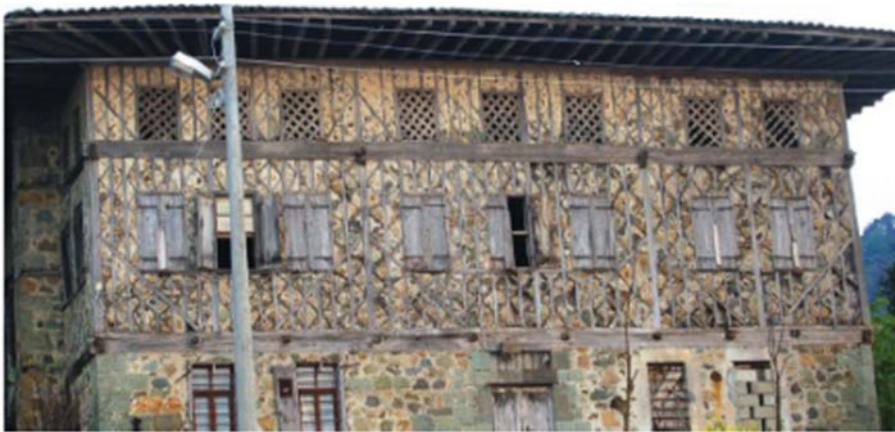
Figure 13. View of a timber structure supported by buttresses to corner posts (Güneş, 2014).
