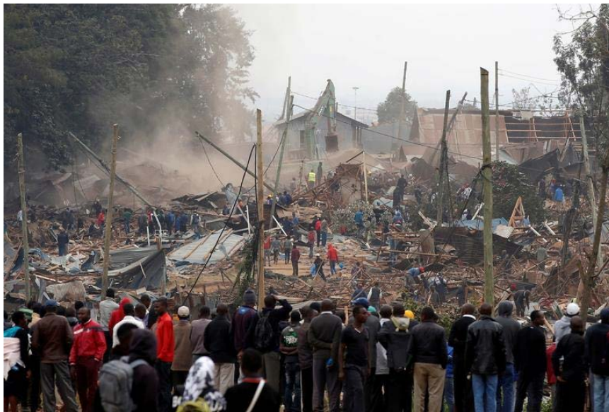
Figure 3. Kibera slum demolition to create room for road construction. (News from Reuters dated 2018)
