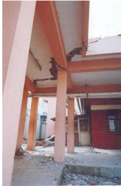
Figure 3. Damage in the re-entrant corner of an L-shaped building (source: Anonymous, 2000, Arslan and Korkmaz 2007)
