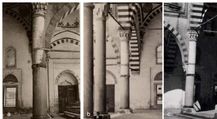
Figure 14. The CL1 column, Selimiye Mosque: a-c) a date between 1913 and 1963 (Source: Ali Saim Ülgen Archive, URL-1)
