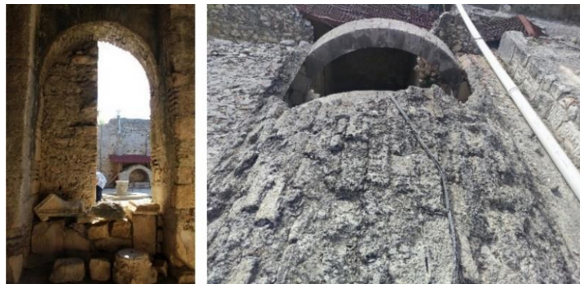
Figure 19. The outer narthex that closes off the western corridor arch and its collapsed vault (AMoCT-PR-4)
