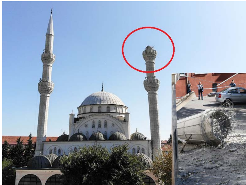
Figure 1. Photo of the collapsed minaret in Avcılar, Istanbul (URL 1)
